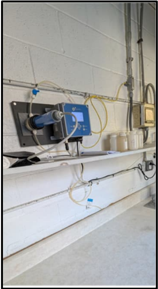
Gully Branch GWTP New Multi parameter pH / chlorine meter
