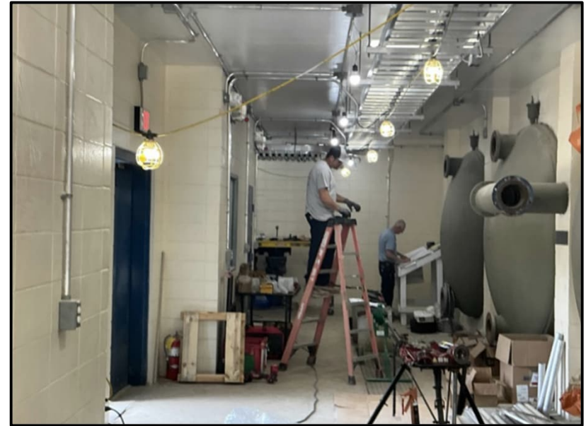
GE GWTP New filter gallery and piping set for real time monitoring and automatic controls
