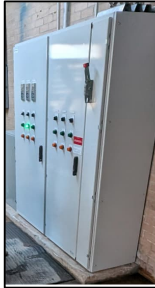
Gully Branch GWTP New MCC and RTU for automatic pump controls
